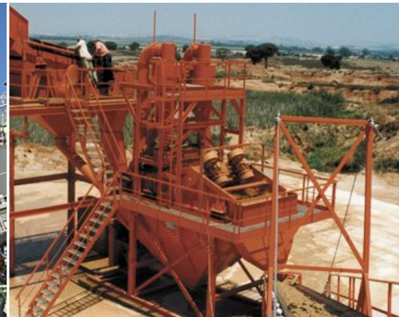
Sand washing (200 tph)
