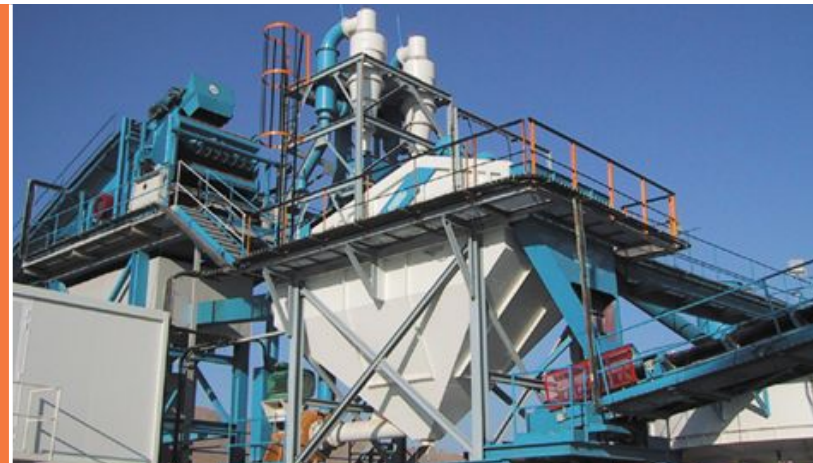
Sand washing (350 tph)
